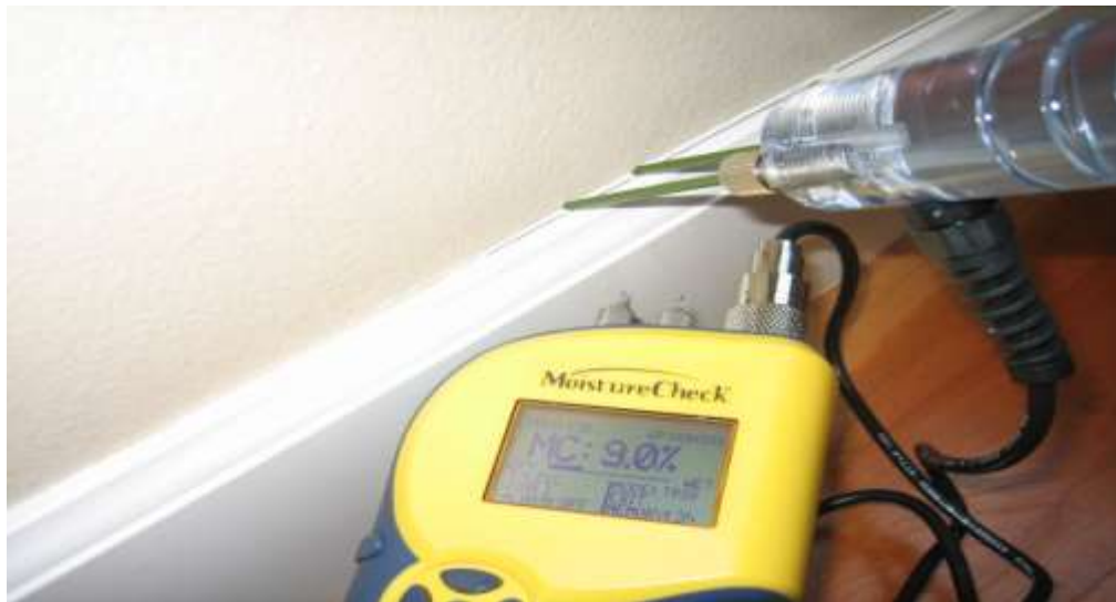
Figure 4: This deep wall probe is inserted directly inside and below, at the sill plate, the probe in the photo above. The 9% MC reading confirms that the moisture from deck rail outside has not entered the wall cavity.
