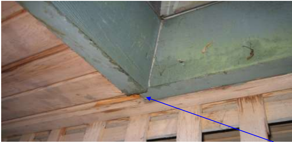
Figure 1: The damaged sheathing material is located directly behind the lowest trim board on the deck structure.
