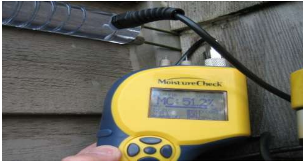
Figure 3: The only area of high moisture content related to the deck rail cap joint was at the lower south side deck. This is the deck with the most exposure to driven rain. Minor damage to the sheathing material was noted in the area.
